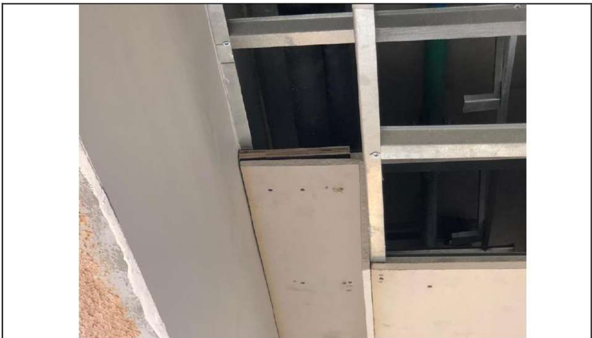
Ply wood to be fixed properly
